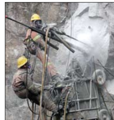
Capilano Suspension Bridge for the construction of an overhanging boardwalk, scalers Mike Talarico and James Haldane drilling and blowing out holes, and working off ropes and spider cage for rock bolting and anchoring to stabilize the cliff face.
