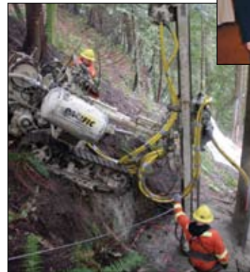
Members Peter Tazelaar operating the winch and brake while Joe Gauvin operates the airtrack controls at the Capilano Suspension Bridge.
