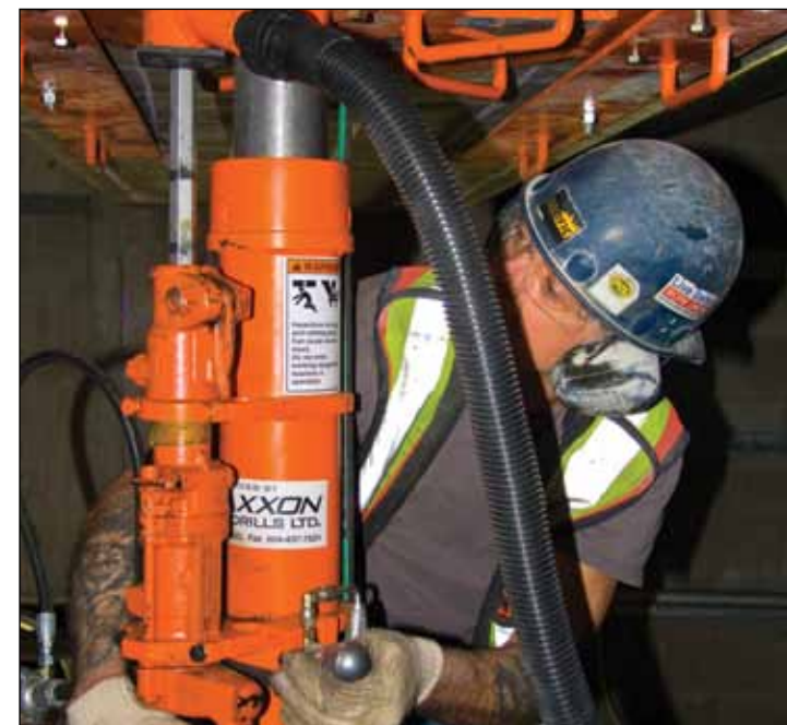
Brian Pearson, cutting & coring division of Traxxon Rock Drill division of Pacific Blasting using the vertical drill under BC Place. Total of 5800 holes, 13/8" holes 16" deep.
