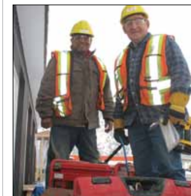
Right Alex Sheloff and Irvine Whitehead working with Aecon loading material on truck deck.
