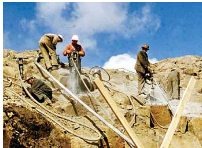
Plugger drilling crew preparing shot rock for dam construction. Photo courtesy of Rio Tinto
